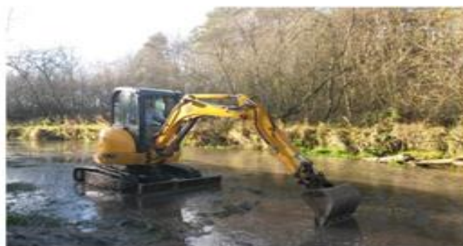
Gravel raking to improve quality for spawning fish. Funded by the Fisheries Improvement Programme
