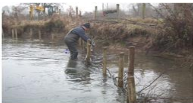
Willow spiling to restore a section of eroded bank. Funded by the Fisheries Improvement Programme
